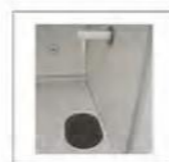
Water Tap & Water Sink
